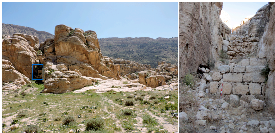
Fig. 9. Dam in Wadi Hirsh (left) and the dam wall (right) detail. Source: Marsal, 2021
