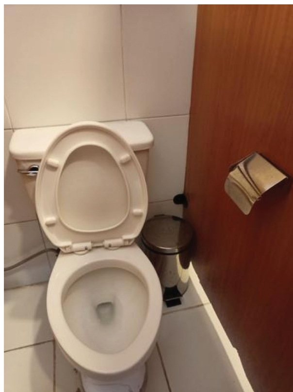
Figure 6. Toilet cubicle with disposal bin but without toilet paper in Manila.
