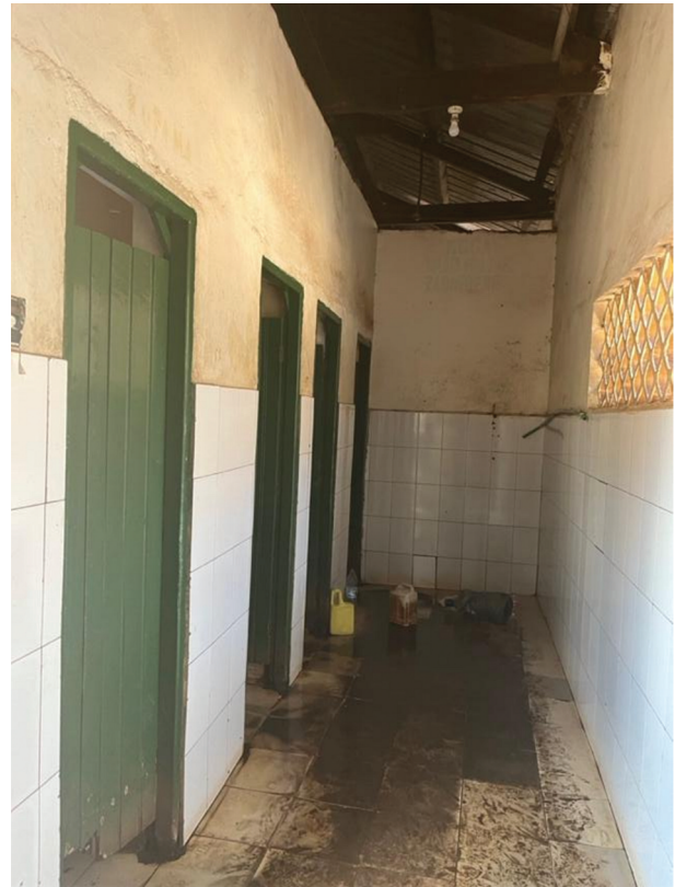
Figure 4. Public toilets inside a transportation facility in Kampala.
