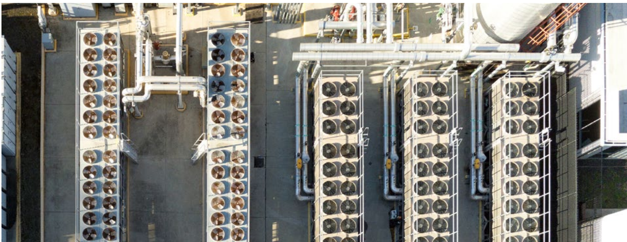
Cooling system at Intel's Mission Campus in Santa Clara, California.
