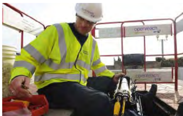
Our fibre network now covers around two thirds of UK premises.
