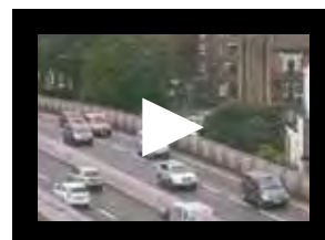
Replacement of the prestressing on a bridge in London. Running time: 2 min 44 s.
