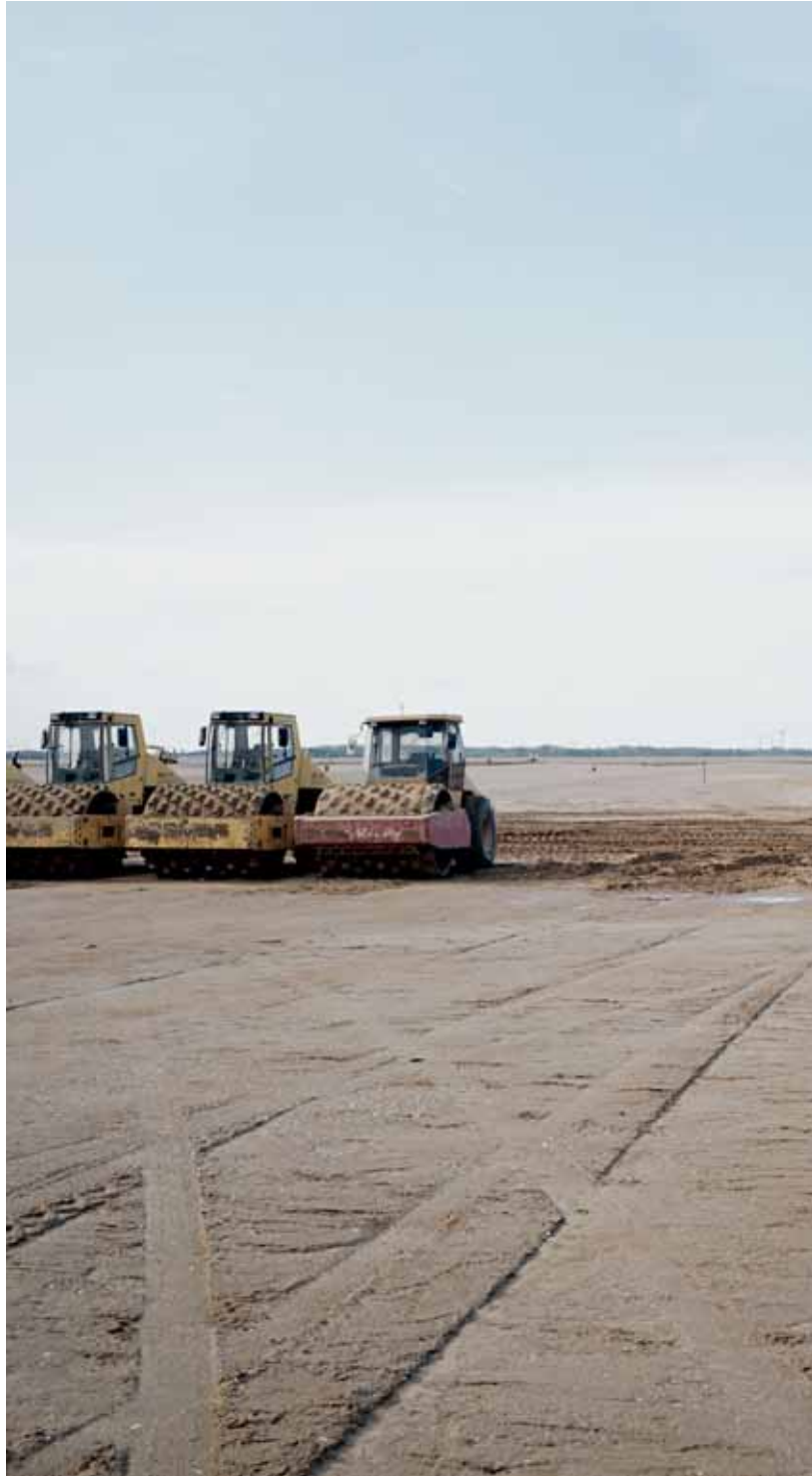
The new location: 208 hectares, to the north of Leipzig. In the late summer of 2001, the site is prepared for construction work. Almost four million cubic metres of earth are moved in order to level out the north-south slope on the property – a volume that is the equivalent of approximately 100,000 truckloads.
