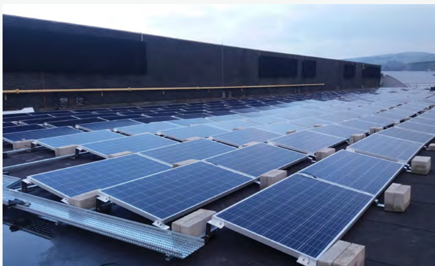
Macclesfield solar panels
