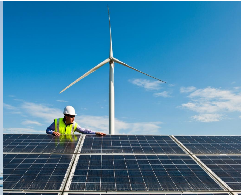
Bollene photovoltaic park, France
