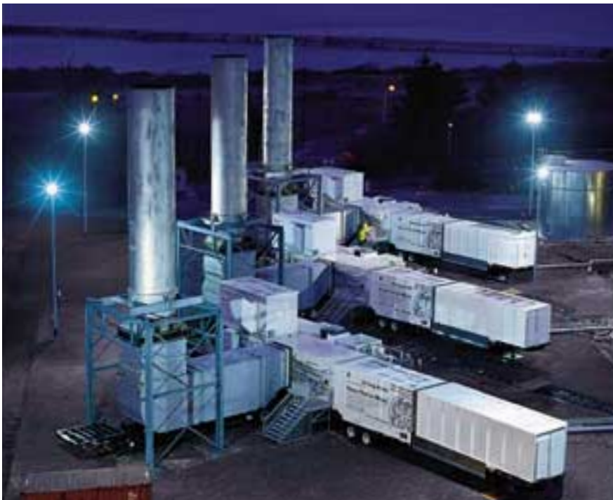
This trailer-mounted Power Plant on Wheels is located in Cork, Ireland. These 22.8 megawatt units are more fuel-efficient and more environmentally friendly and occupy less space than other temporary power solutions.
