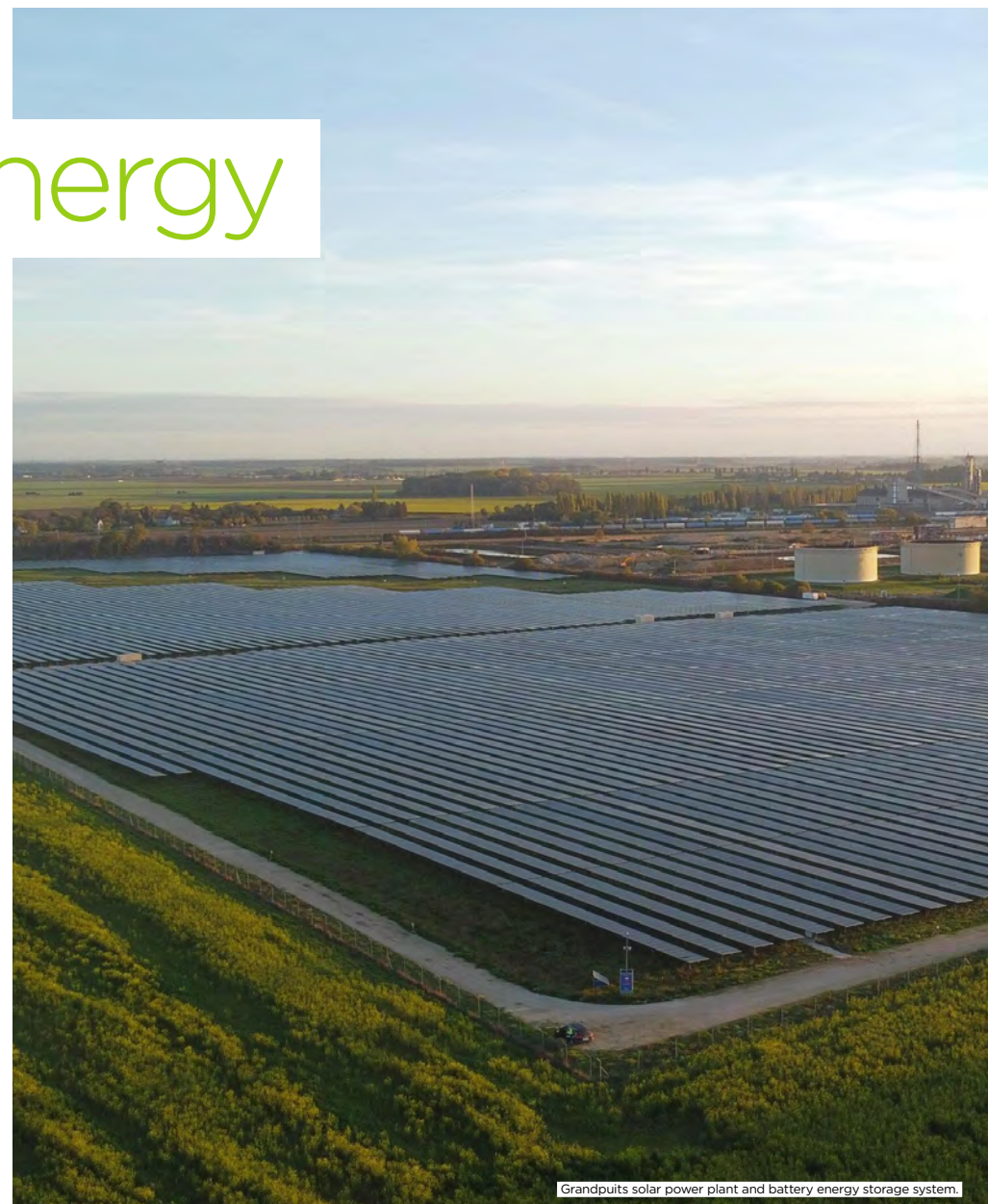
Grandpuits solar power plant and battery energy storage system.
