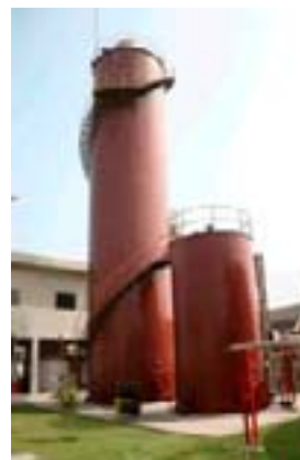
Wastewater Treatment Plant at AmBev's Huachipa, Plant near Lima, Peru.
