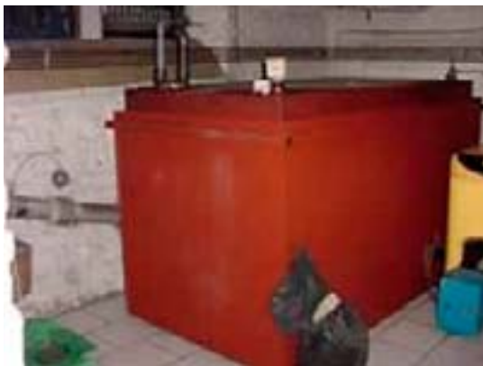
An upgraded fuel storage installation in a private house in the Jupille community in Belgium.
