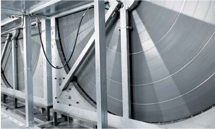
above -- Energy efficiency in the Leipzig plant: Exhaust air from the factory halls is used for heat recovery with a total of 20 heat wheels.
