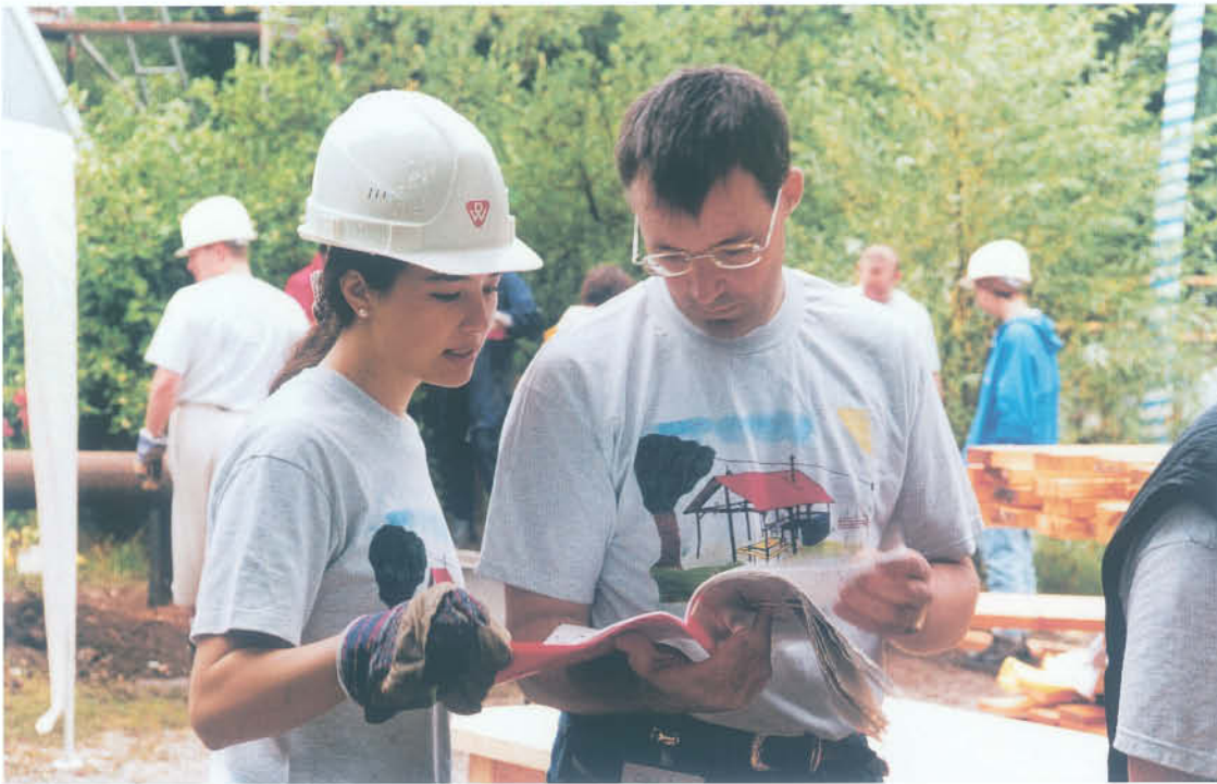
The employees at Siemens Corporate Consulting were determined to do more than just pass on charitable donations to unknown recipients. By harnessing their various skills, they were able to renovate a youth center in the Munich area of Hasenberg.
