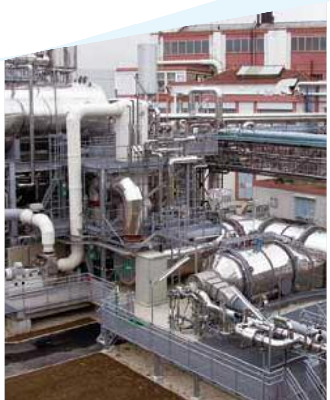
Thermal oxidation treatment facility for Volatile Organic Compounds (VOCs) at the Vitry Production Center
