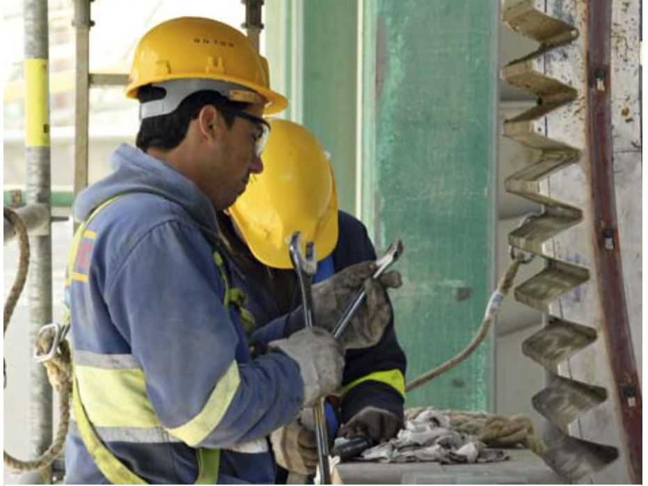
Construction of the Tanger plant, Morocco. Work at height. © DR Lafarge Medialibrary
