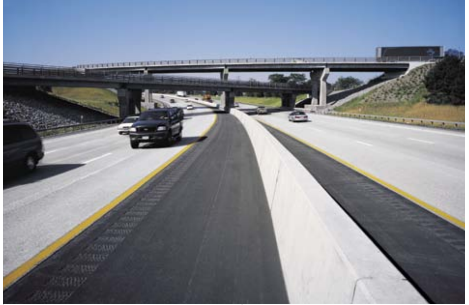
Recycled asphalt products help spare virgin aggregates. Concrete Highways, Buffalo/Rochester, New York, USA. © Lafarge Medialibrary - K.C. Kratt - GPA - New York State Department of Transportation Region 4 - Authority New York State Thruway - Transportation Parson - Ressel Howard (architect)
