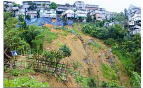
Earthquake-prone house in sloping terrain in Aizawl, a city with 300,000 inhabitants in north-east India.
