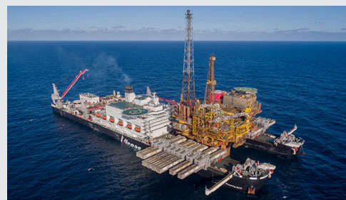
The Brent Delta platform weighs the same as 2,000 London buses and is as high as the London Eye.
