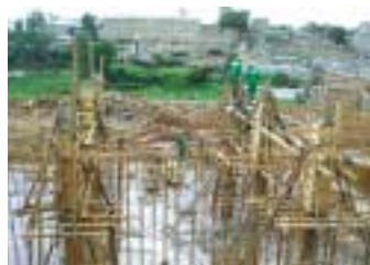
The new brewery effluent treatment plant in Nairobi, Kenya will reduce BOD emissions by 80 per cent. The project will be complete in 2005 and cost £2.16m.
