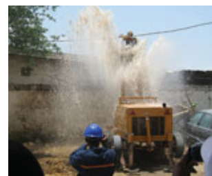
Projects in Cameroon, like this one at Kassalafarm, delivered water supplies to 116,400 people in four communities
