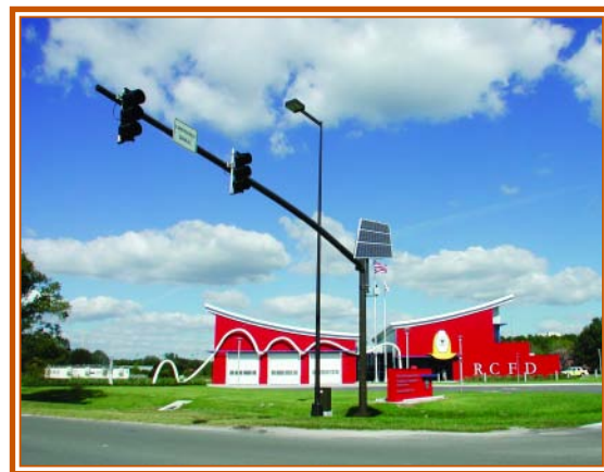
A solar-powered traffic light installed in front of a new firehouse at the Walt Disney World Resort will benefit both the environment and the bottom line.
