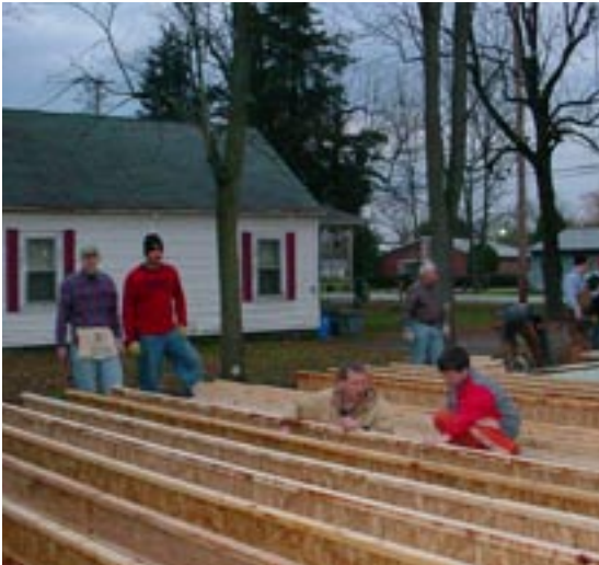
GM's Powertrain Defiance Professional Managers Network builds a Habitat for Humanity House in Defiance, Ohio.
