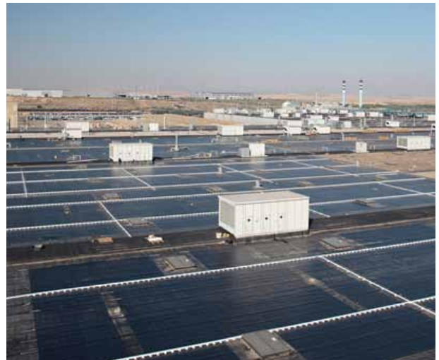
Solar panels installed on rooftops provide renewable energy to those facilities.
