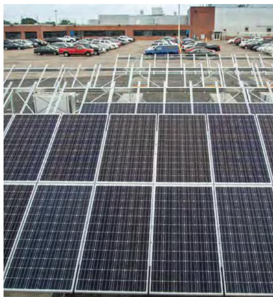
A new 800-kilowatt solar array at the Warren Transmission Operations is GM’s largest solar installation in Michigan.
