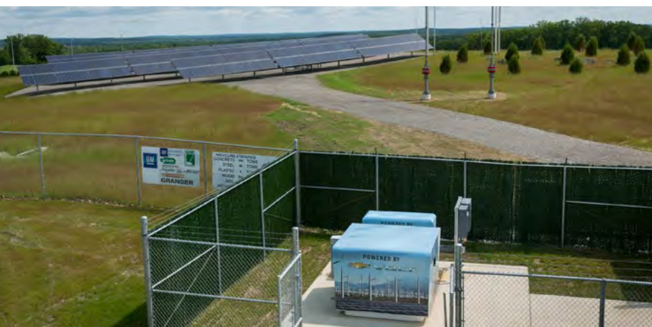
Used Chevrolet Volt batteries are helping keep the lights on at the new General Motors Enterprise Data Center at its Milford Proving Ground in Milford, Michigan. Five Volt batteries work with an adjacent solar array and two wind turbines to help supply power to the data center's administrative offices.
