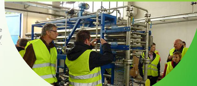
E4WATER consortium members observe the breakthrough water recycling technology at our Rakona, Czech Republic, site.
