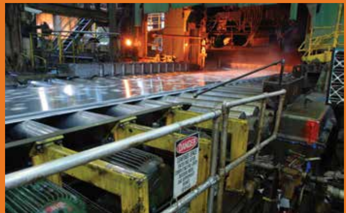
Coolant spray on the hot reversing mill
