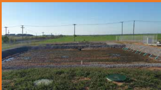
NEWT system at Wichita Falls
