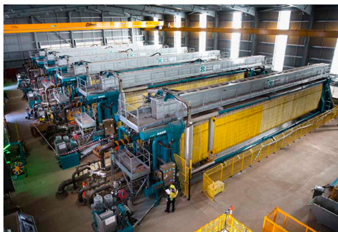
Pinjarra filtration system
