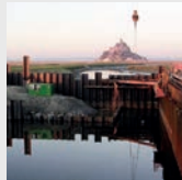
ArcelorMittal's sheet pile solutions are helping to save Mont St Michel in France which is gradually becoming attached to the coast by the accumulation of sand. The project aims to retain water from the river Cuesnon, and to release it like a flush to carry away the sand surrounding the island.
