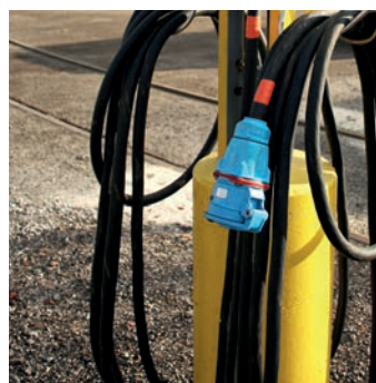
Cleveland railroad's external power stations: when not in use, locomotives plug in to these new external power stations, saving money in fuel costs and reducing diesel emissions.
