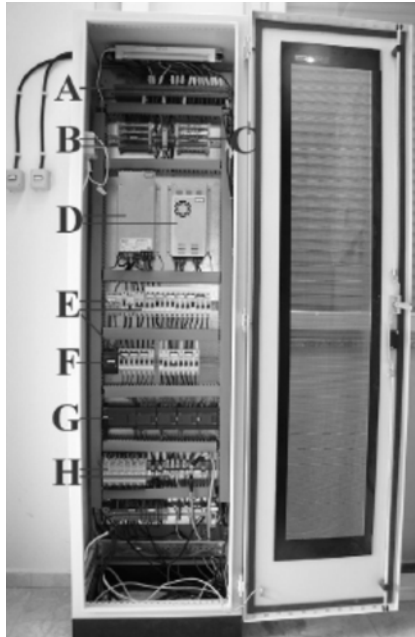
Fig. 9. DC power distribution box.
