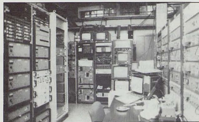
Interior del Centre Emissor del Tibidabo
