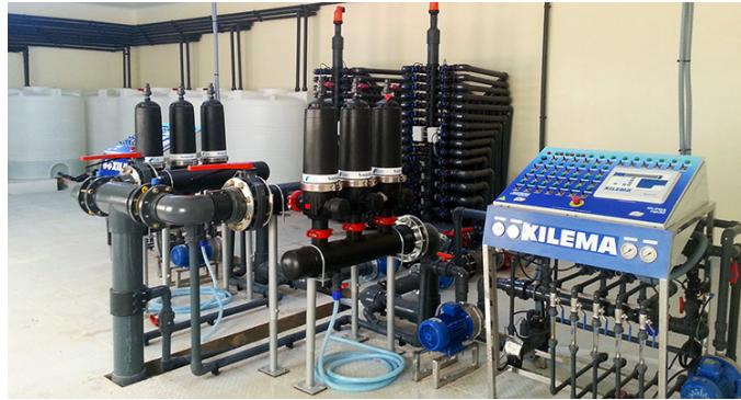
Figure 33: Irrigation Head Source: Novagric
