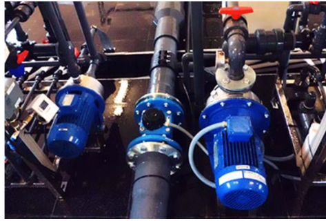
Figure 36: Irrigation Pumps Source: Novagric
