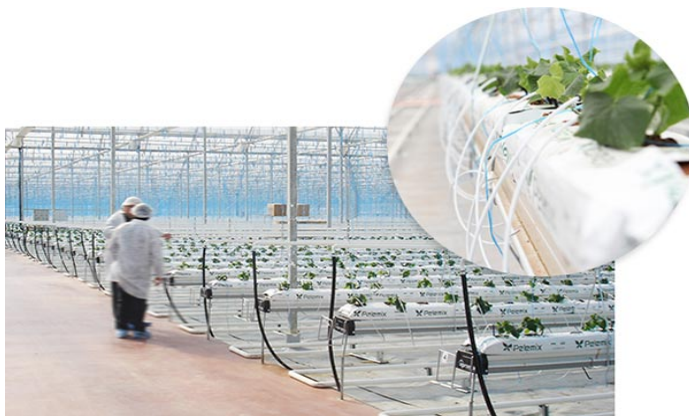
Figure 48: a Drip System Installation Source: Novagric
